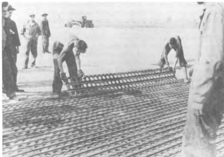
Laying a pierced steel plank runway: the "Marston mat." ( U.S. Army Corps of Engineers. )
